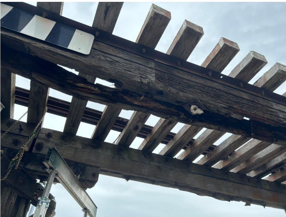
Photo 2: Split in bottom beam
