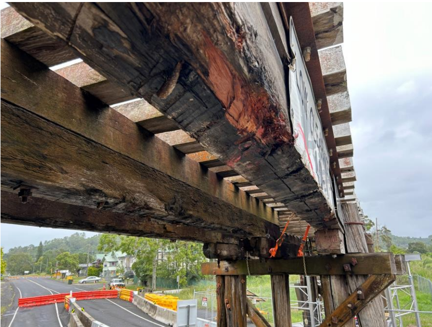
Photo 2: corbel displaced (far end) and damage to side of girder.
