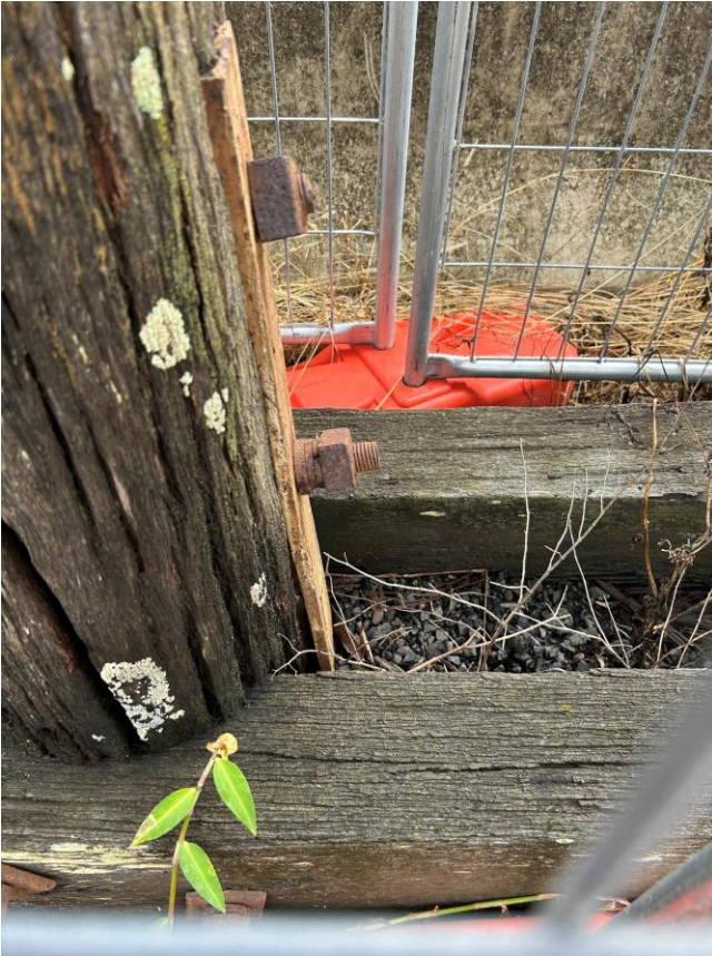
Photo 3: pier 4 column appears to be displaced in relation to plate
