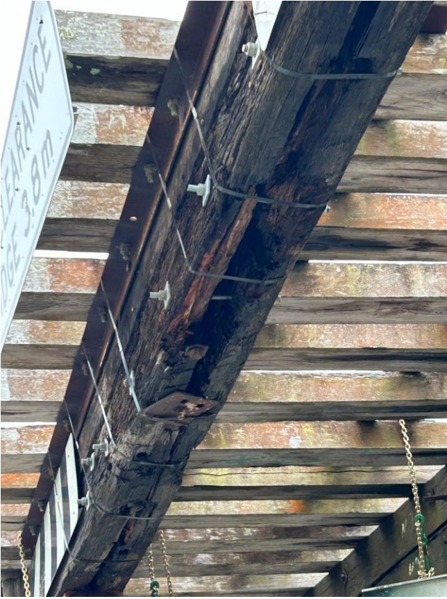
Photo 1: Split in bottom beam from impact in Jan 2024
