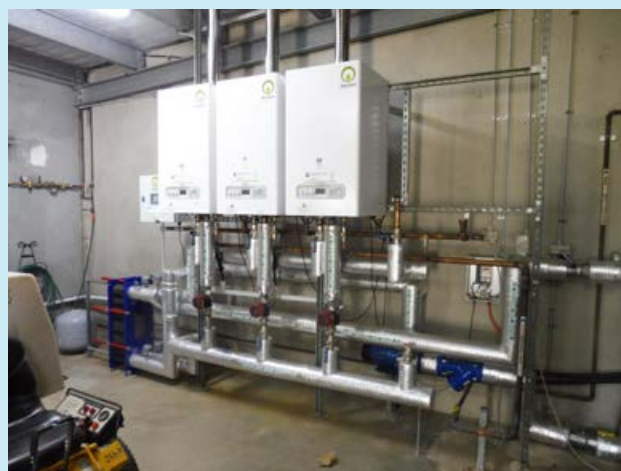
Figure 2 New high efficient condensing boilers (ESBS Pty Ltd)
