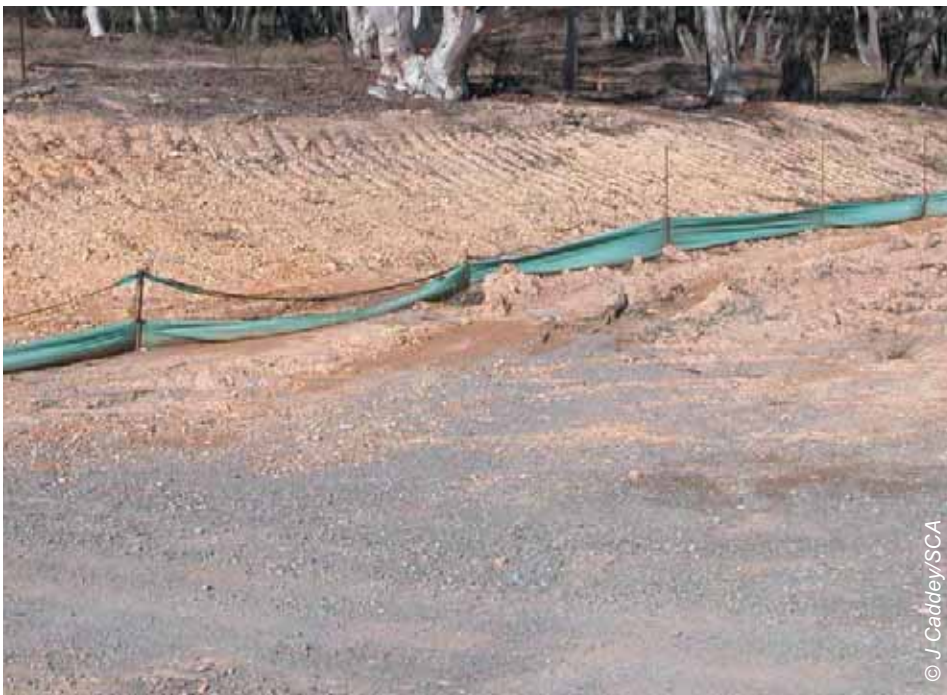
Figure 6.6 Erosion and sediment controls are only as effective as their maintenance
