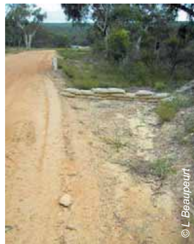
Figure 6.4 A sandbag sediment trap with a spillway in the outlet of a table drain
