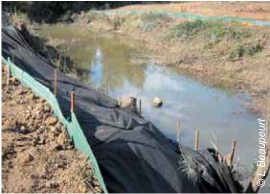
Figure 6.8 Temporary erosion and sediment control measures along a creek
