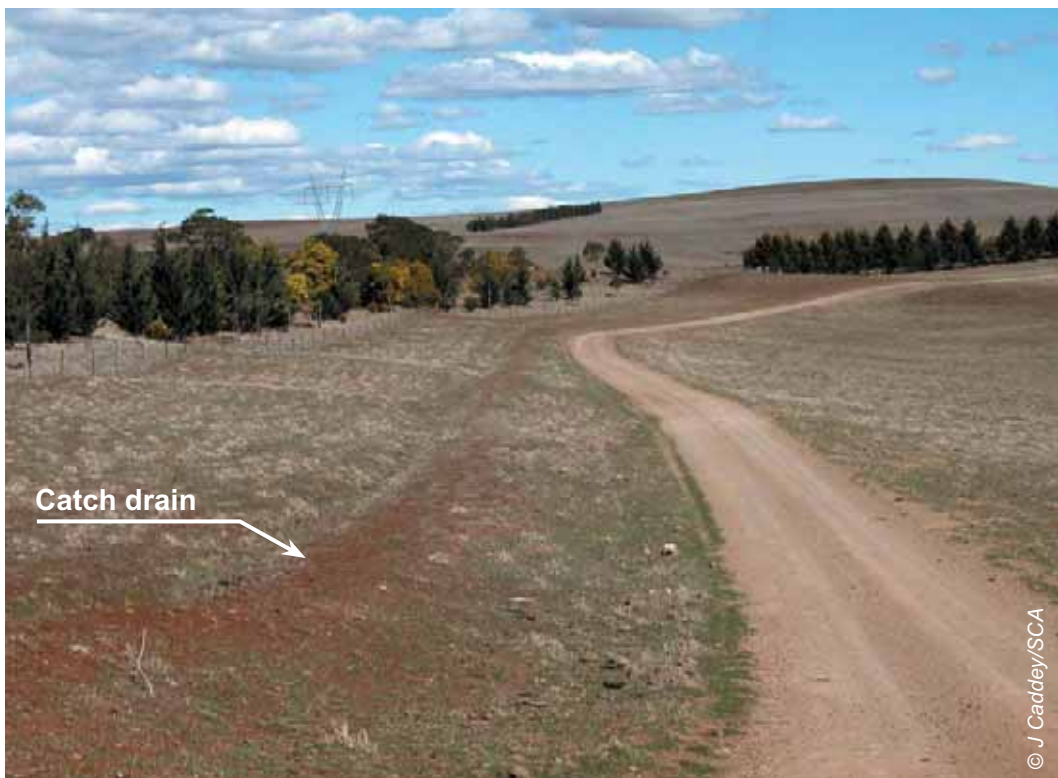
Figure 5.11 The lining of a catch drain should be selected to suit the size of the catchment above and slope steepness
