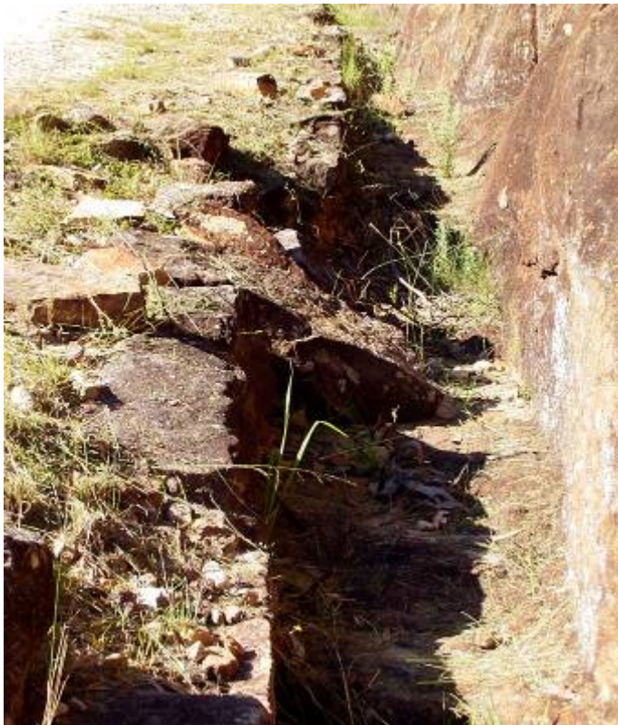
Figure 30 Displaced kerb stones that have fallen into the side drain, reducing its capacity and risking erosion of the road pavement.
