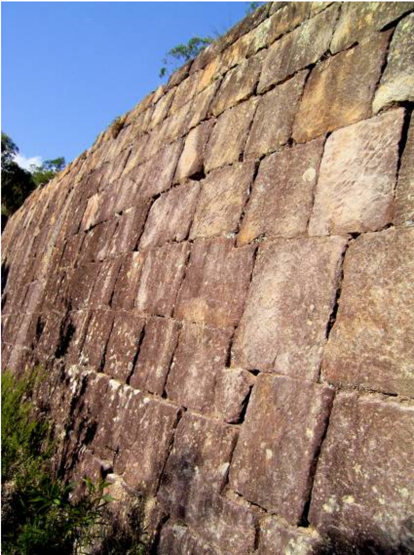
Figure 3 Remarkable quality drystone retaining walls are a feature of the Devine's Hill ascent (Precinct 1).
