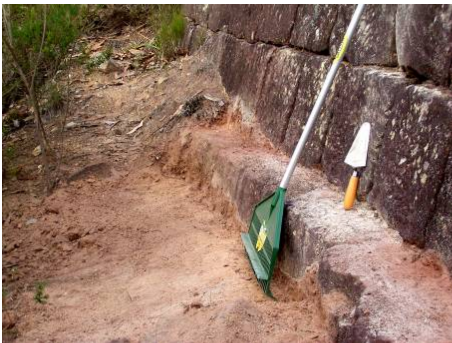
Figure 26 Accumulated sediment is removed from the base of retaining walls using a strong plastic rake and a round-headed (gauging) trowel. The trowel is used to free root-bound earth from the stonework. The basal course of stone is left half buried to protect it from erosion.
