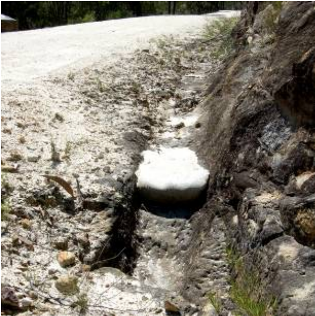
Figure 27 Sandbagging of drain to catch silt run off from recent (2006) resurfacing of portions of the Devine's Hill ascent. This silt is collected and disposed of. Sandbags should be removed once the amount of run off has stabilised. Like the culvert in Figure 4 this one is missing its original entrance cover: recesses in the sandstone bedrock on either side show where it was fitted.
