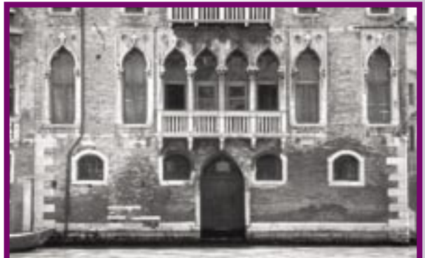
Fig 35. Capillary rise of sea water in an old building in Venice (Reference 22)
