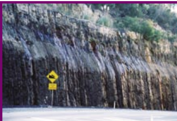
Fig 9. A raised ground water level may be evident in road cuttings after periods of abundant rainfall
