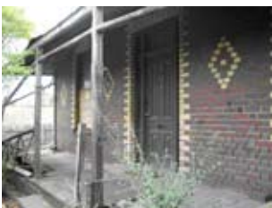
1883 brick cottage, before and after restoration. Images courtesy Ray and Jennifer Bantow.
